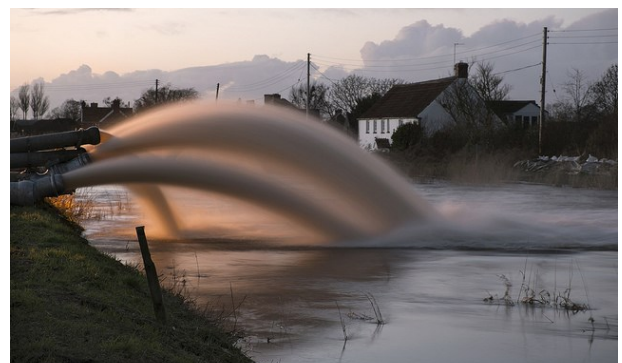
Emergency pumps on the Paret, by Noel Jenkins , CC BY-SA 2.0
